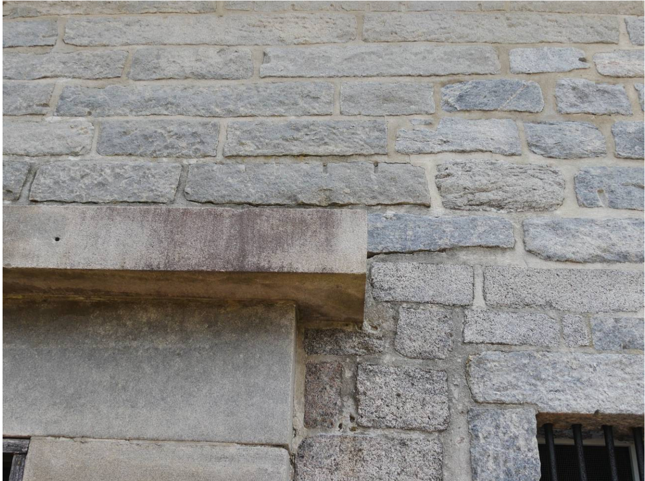
Figure 6 – Close-up of the stonework on the west side. The stonework of the entrance is in the lower left of the photo.
