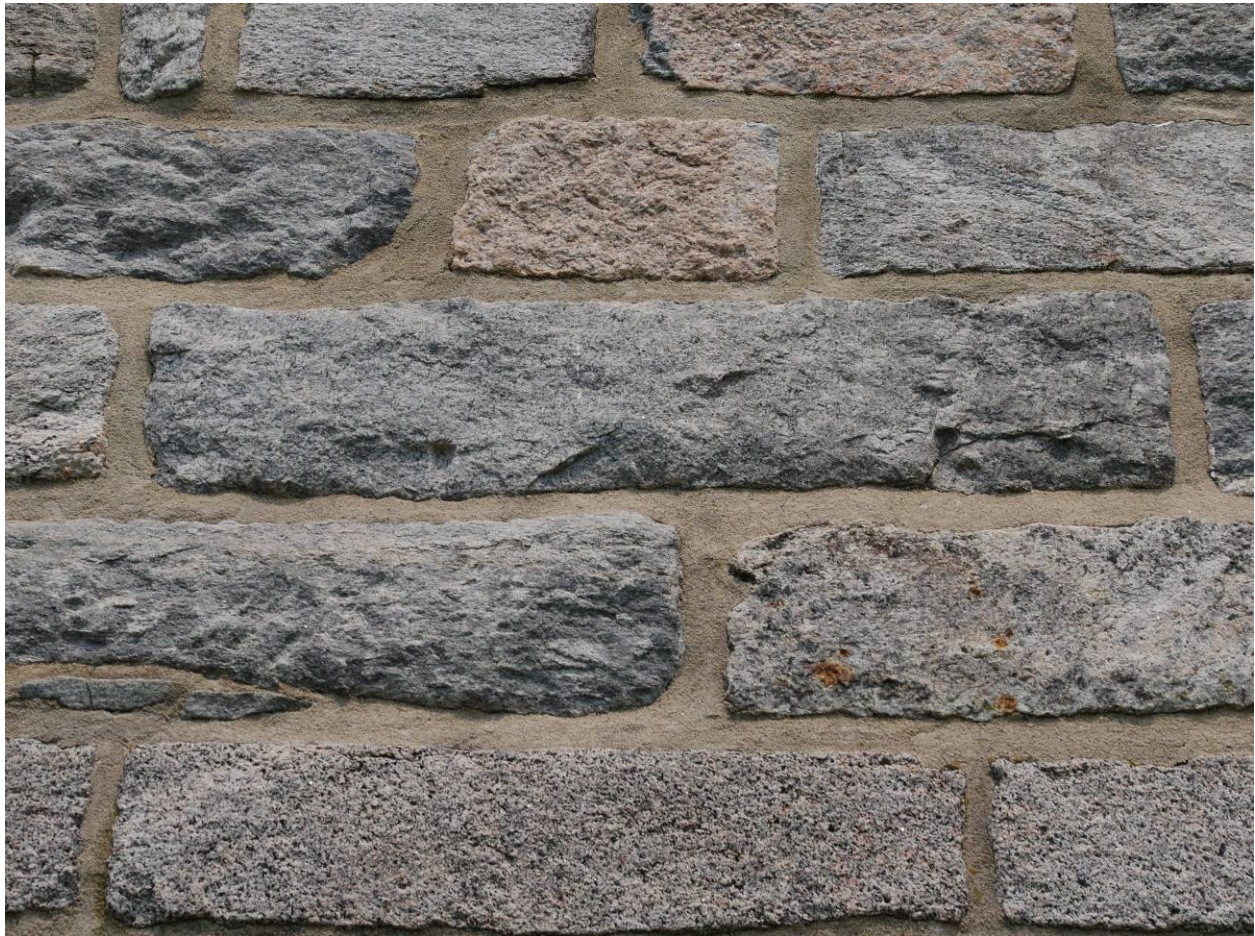
Figure 4 – The bottom layer in this photo is the semi-smooth pinkish-tan color of the original 1794 block house stonework. The rough stones in the three layers above of it are part of 2 nd phase which involved repairs and additions made to the building.
