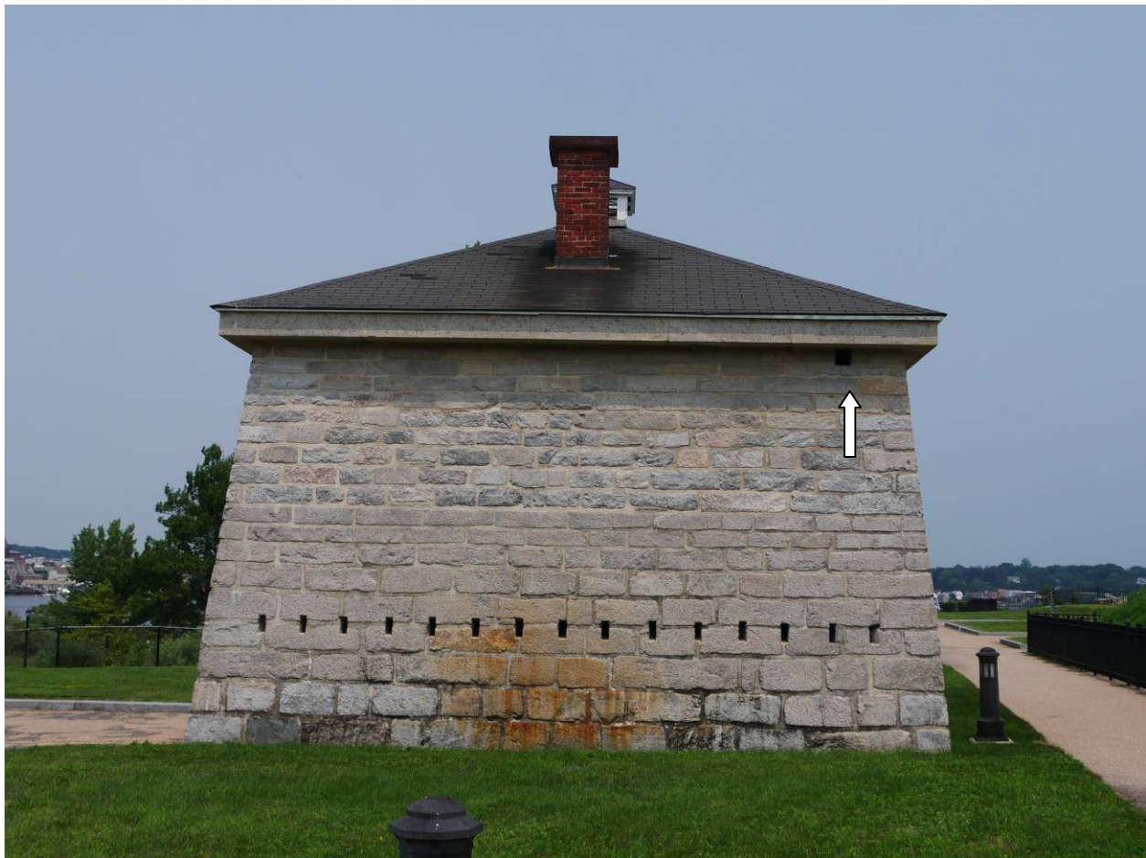
Figure 2 – South side of block house with fifteen gun ports and a vent hole in the upper right below the stone eave of the roof (indicated by the arrow).
