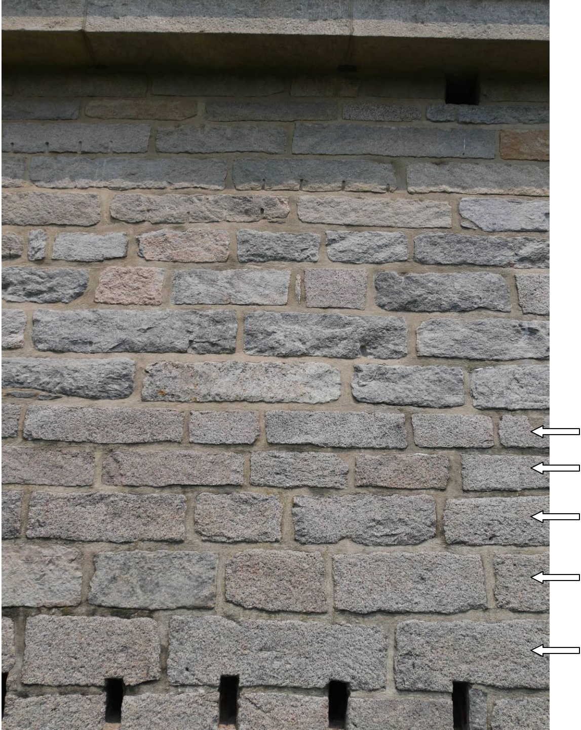
Figure 3 – Close-up of south wall. Note the uniform color (pinkish-tan) and surface texture (semi-smooth) of the stones in the lower half of photo (arrows). It is different from the blue-gray color and rough surface texture of the stones in the layers above it.
