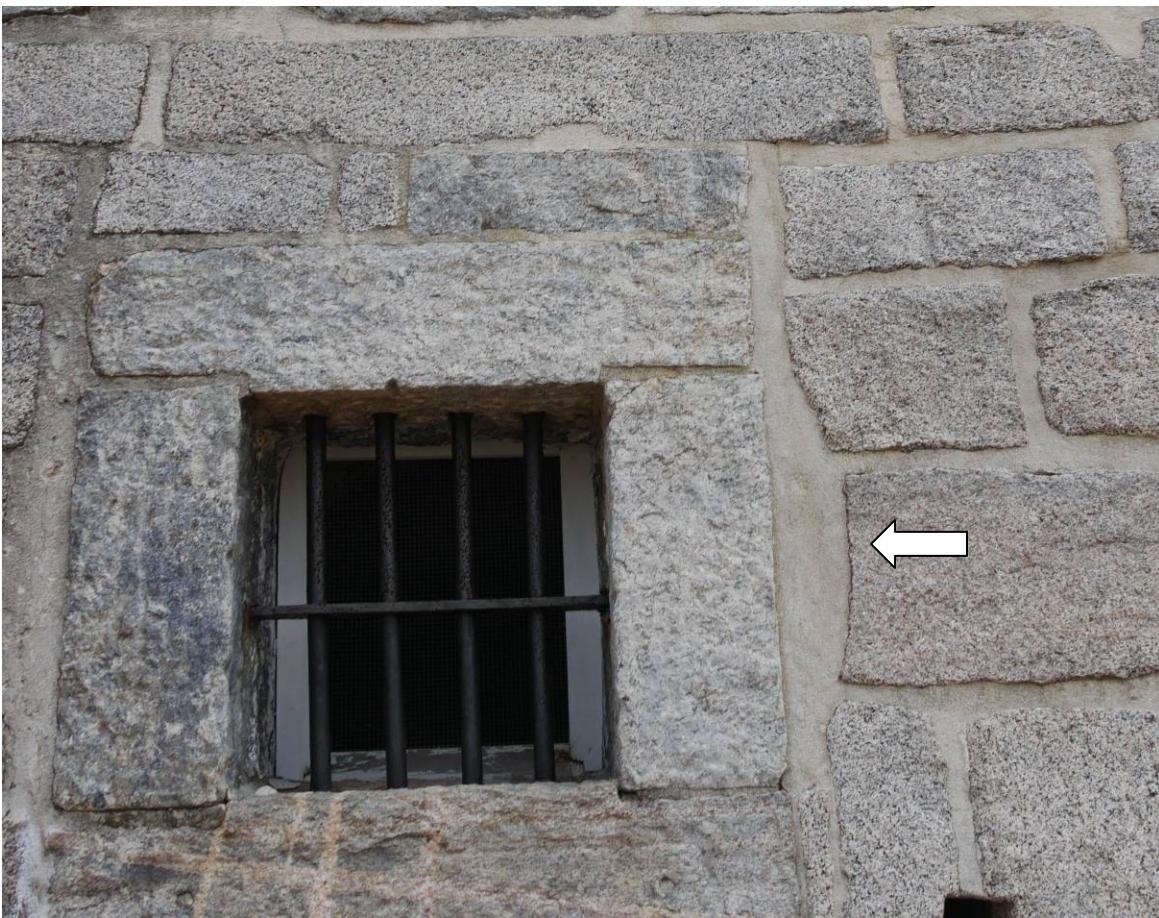
Figure 7 – This photos show details of the window on the right side of the entrance. The arrow points to crescent shape cut to accommodate the original round windows. There is a matching crescent shape on the left side of the window.
