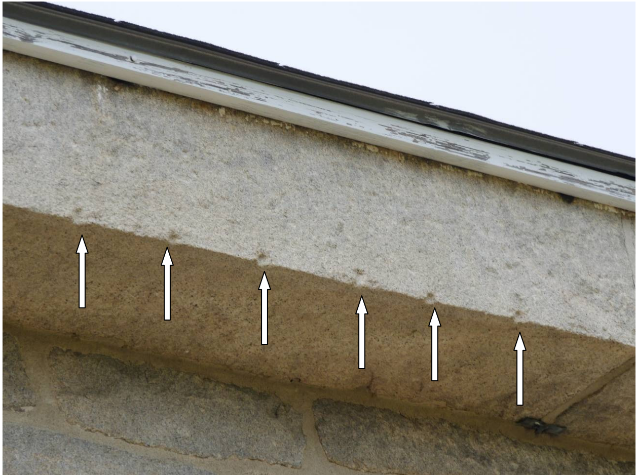
Figure 5 – The roof eave stone on the east side of the block house has the same color and smooth finish of the stones in Fort Trumbull. Remnants of drill holes from the commercial plug and feather method of splitting the stone are visible and indicated by arrows. This phase of repairs and renovations dates from the 1840s.
