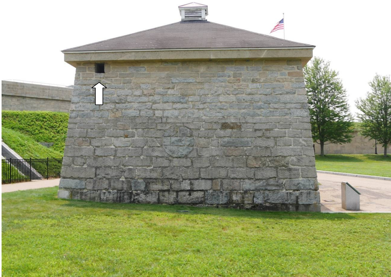
Figure 8 – Overall view of north wall. Arrow indicates vent near top of roof under the stone eave.
