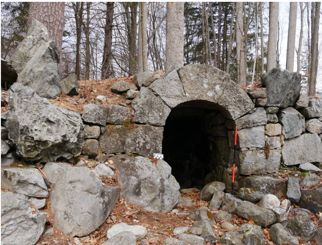
Figure 9 – Plug and feather method quarried granite arch entrance of the south grotto. Another one of the sculpted (differentially weathered) stones is seen to the left of the entrance.
