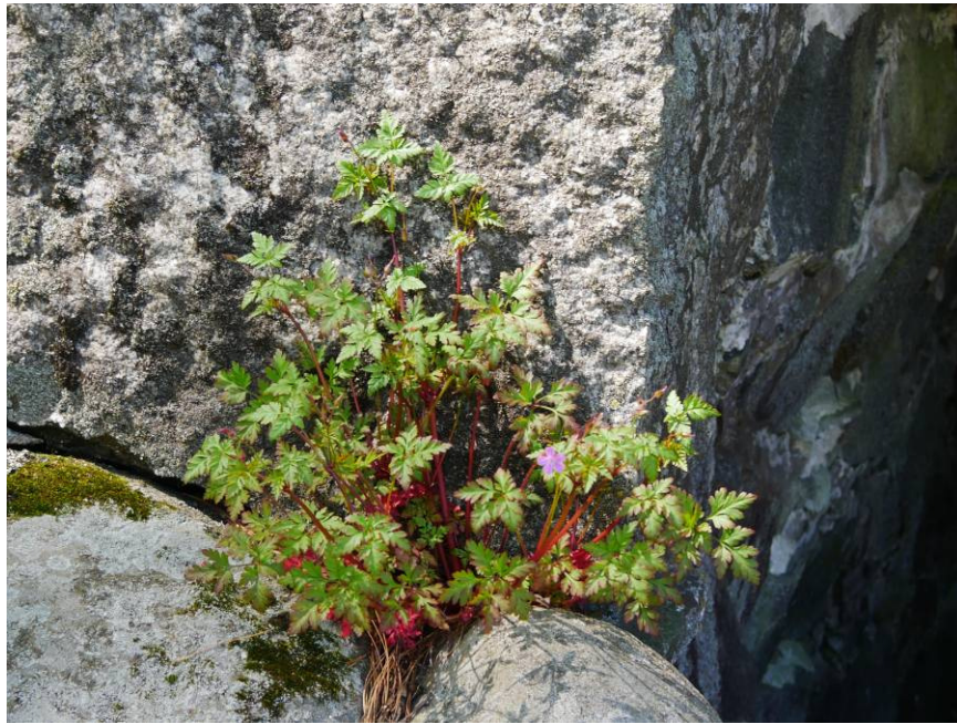
Figure 18 – Flower growing out of the arch stonework of the south grotto.
