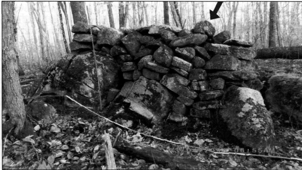
Figure 4. This pre-1800 cairn exhibits slanted stone stacks that create vertical joints (#1365, West Side – Jonathan Foster Farm).
