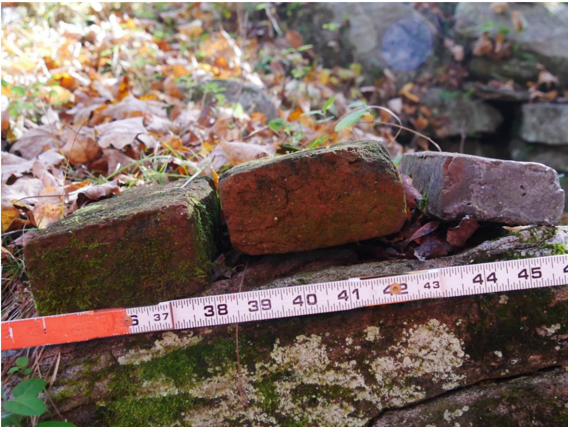
Figure 9 - Bricks placed on top of the wall of the cellar entry (side view)
