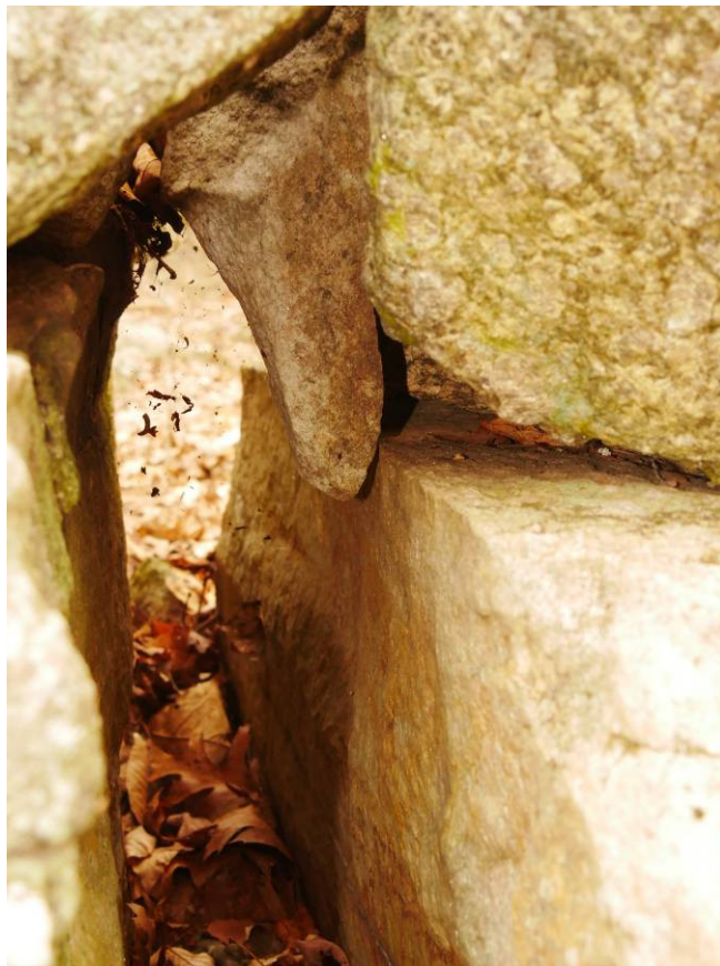
Figure 50 – “Tongue” feature protruding downward
