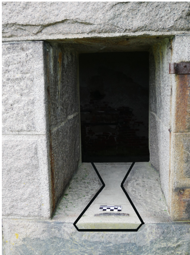
Figure 13 – The standard size gun port was widened by splitting off and chiseling the angled out sections of the stone blocks on both sides. Hourglass area (outlined) was filled with cement.
