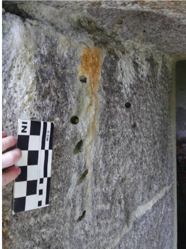
Figure 14 – Drill holes from the process of widening the gun port. No effort was made to erase the marks.
