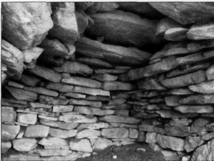
Figure 32. Interior view of the chamber in the Hoffman Evergreen Preserve, Stonington, CT. (Photo by Ted Hendrickson, used with permission.)
