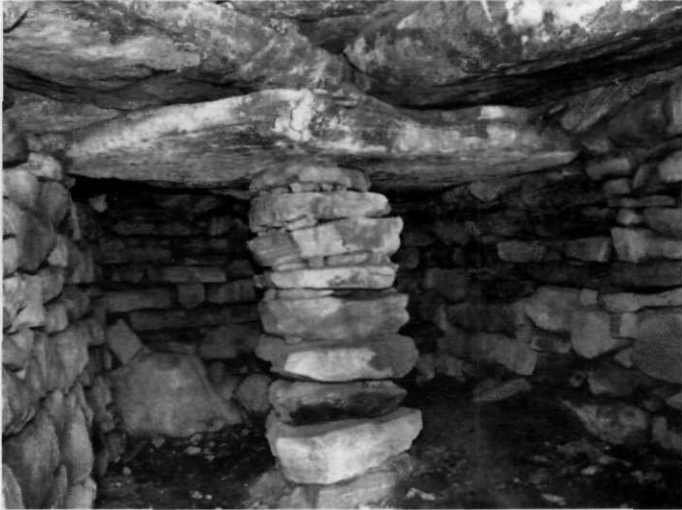
Figure 16. This root cellar has a rectangular room, straight vertical flat faced walls, and square corners. The stone support column is unusual but has been used in some American barns. Ledyard, CT (Photo courtesy of Ted Hendrickson).
