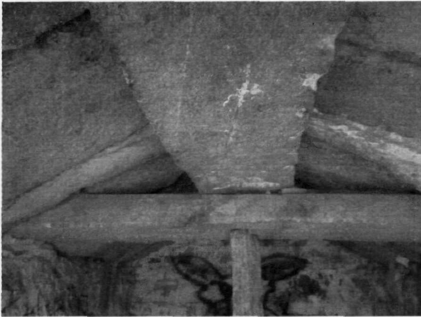
Figure 3. Interior view of the Westford root cellar. The rectangular interior room is covered with a gable roof made from quarried stones supported by a stone ridge beam. (Photo courtesy of David Brody).
