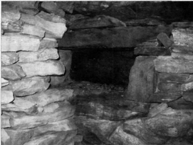
Figure 30. Interior niche in the rear wall of a root cellar. The left hand wall is a 20 th century addition that divided the original room into two sections. North Grosvenordale, CT. (Photo courtesy of Chris Pittman.)
