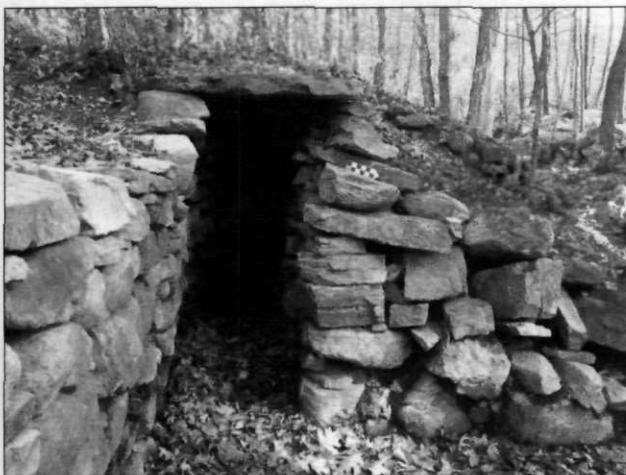
Figure 26. The upper 1/3 of the right wall leans outward. This appears to be an intentional feature rather than structural failure. Stone Chamber, Webster, MA.
