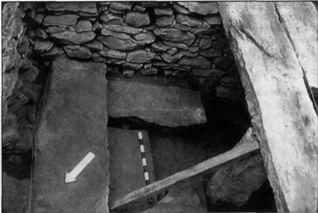
Figure 1. This circa 1823 root cellar was covered with a roof constructed of 14.5 foot long quarried stone slabs (now partially collapsed). Phoenixville, Eastford, CT (Photo used with permission of Old Sturbridge Village (P.83 VIIA Slide #27 Sept. '83).
