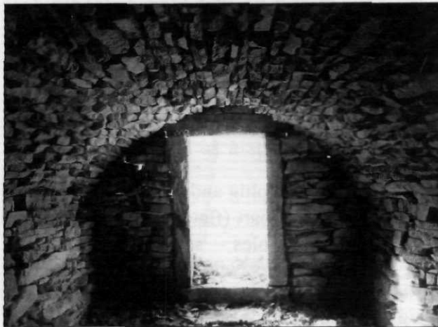
Figure 18. Interior view of the root cellar's stone arch roof made from flat stones. Thompson, CT.
