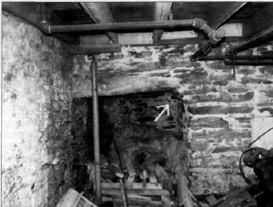
Figure 8. On the right side, two layers of corbelled stones were used to support the stone slab which was not quite long enough to span the whole distance. 1791 John Park House, Ayer, MA.
